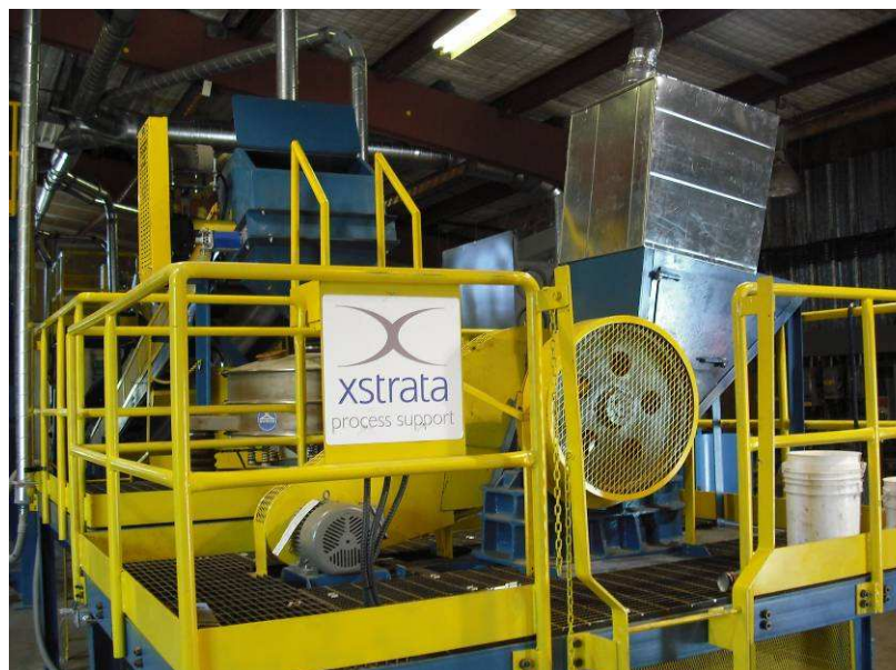
Ready to Rock: View of the primary jaw crusher and secondary screen platforms of XPS' new continuous crushing and blending plant.
